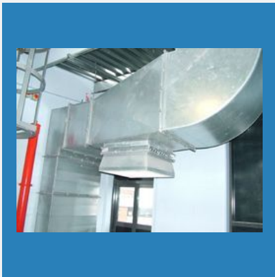
Smoke Exhaust System
