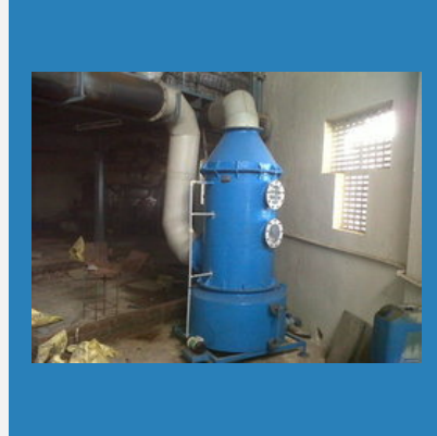
Acid Fume Scrubber
