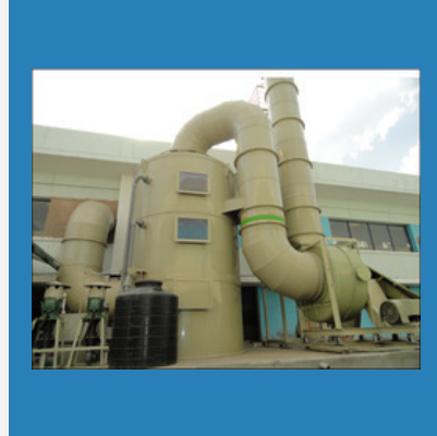
Fume Extraction System
